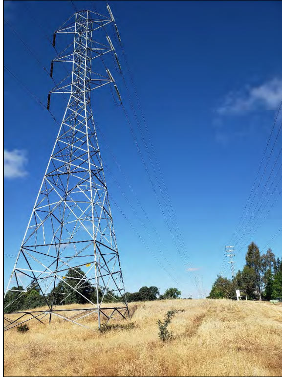
Figure 8. Overview: SV-001, SMUD 230kV transmission line; Diamond Oaks Road, right (view west, June 14, 2021).
