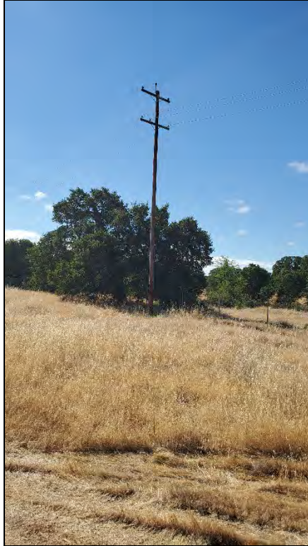
Figure 9. Overview: SV-002, SMUD 115kV distribution line (view southwest, June 14, 2021).
